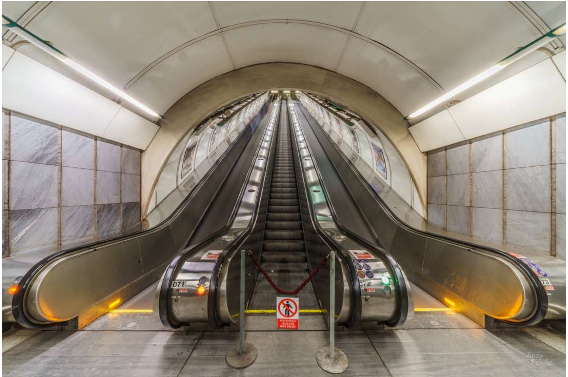
14 - out of order... the station was down to two operating escalators.
